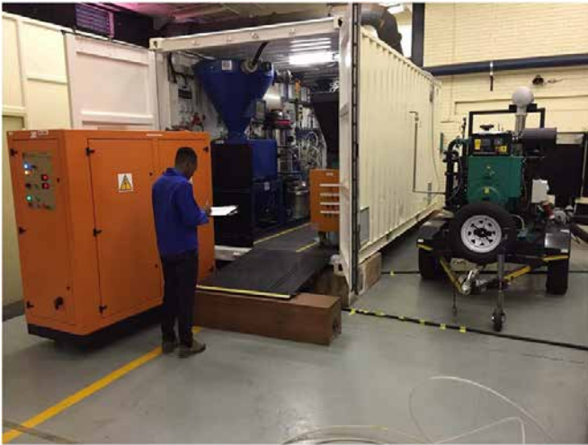
Figure 29. Containerized plasma waste to energy system.
